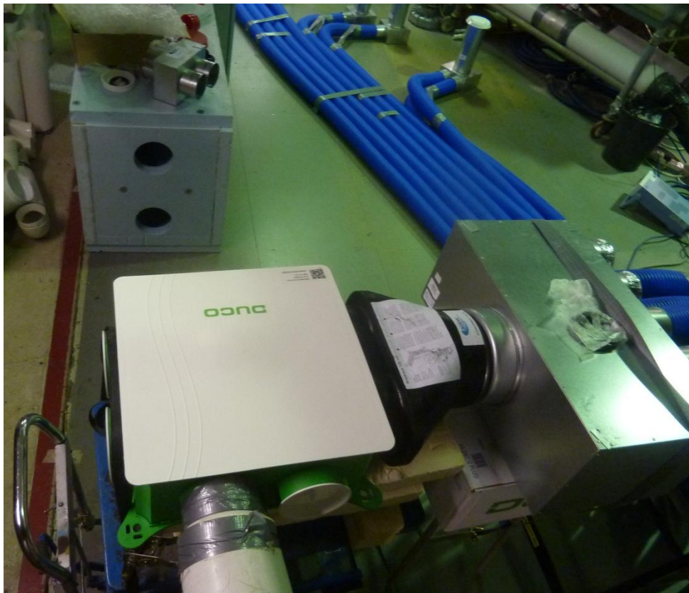
Figure 3 Semi-Rigid duct and plenum installed on MEV unit.
