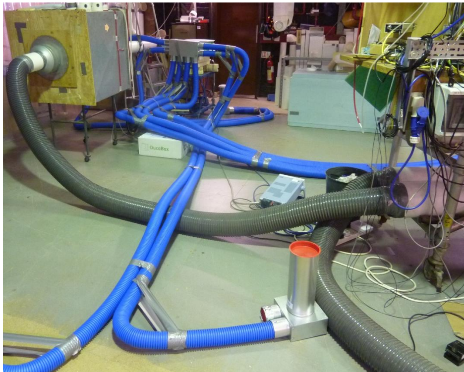
Figure 3 Semi-Rigid duct and plenum installed on MEV unit.
